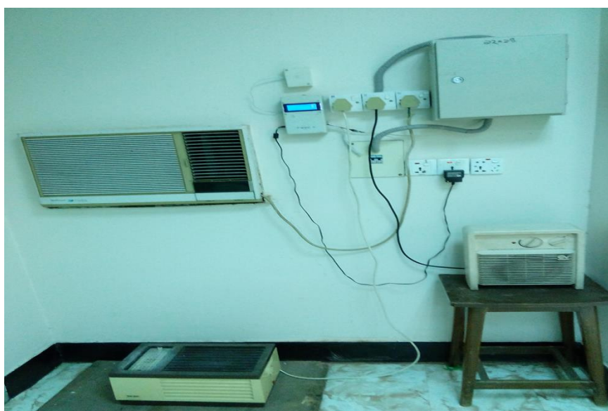
Figure 3.2.4: Temperature (T) and Relative humidity (RH) control panel in Insectary
